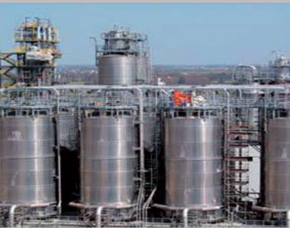
Basell Orlen Polyolefins is recognized for innovations and advanced technologies in its production plants and logistics platform in Poland (Plock).
